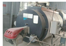
■ Air supply fan for boiler
