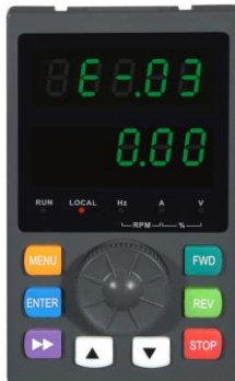
Fig. 4-5 Fault alarm display state
